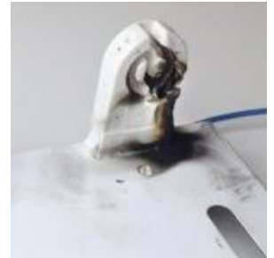
Blade type socket damaged by arc flash
