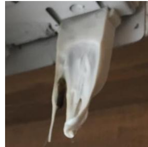
Blade type socket damaged by overheating
